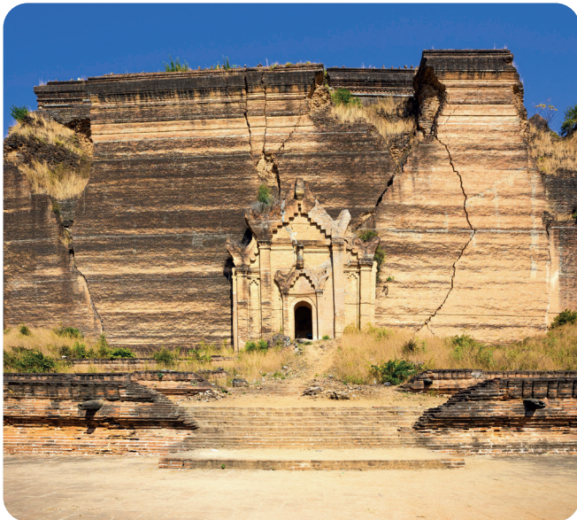
Impact of earthquake in Mingun Pahtodawgyi Temple
